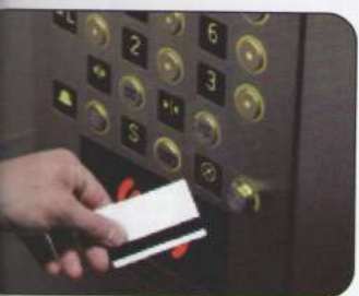
Access Control for Lift
