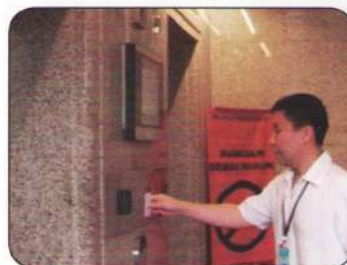
Access Control In Lift
